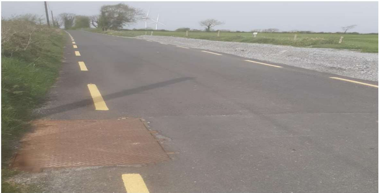
Image 1.4: Example of a Reinstated Road Over a Joint Bay (Darker Asphalt) with the C2 Chamber Cover Visible
